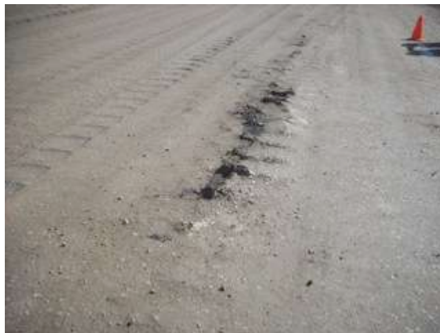
Figure 1. Deformation of the existing slag gravel wearing course.
